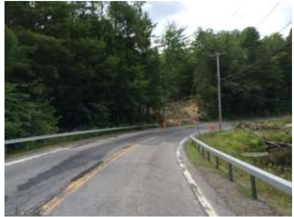
At washout near Big Brook View southwest
