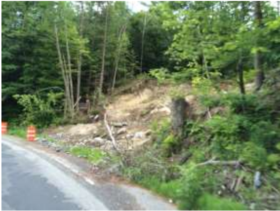
At washout near Big Brook View south
