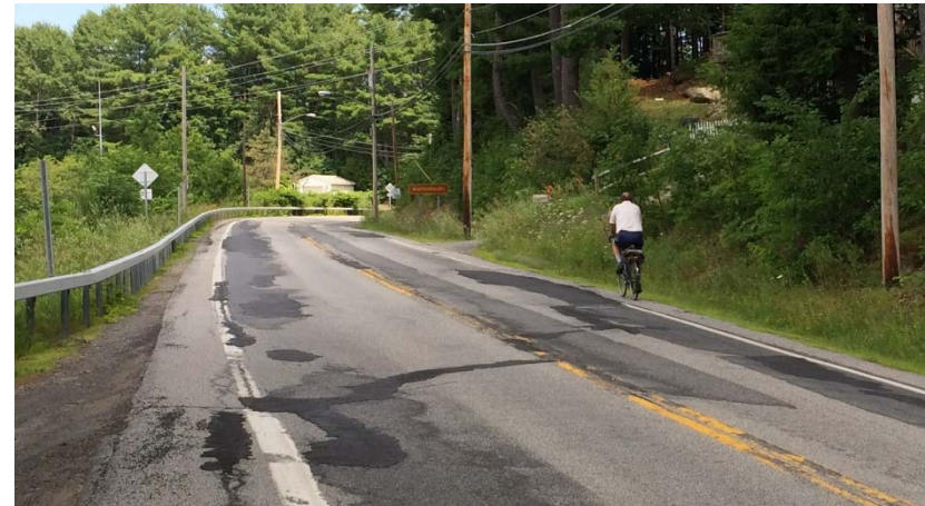
Narrow and poor road shoulder conditions along River Street can deter cycling and can contribute to a number of safety related concerns
