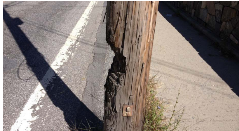
Evidence of vehicle and/or snow plow impacts can be seen on several utility poles within the corridor. Other utility poles are considerably closer to the travel lane.
